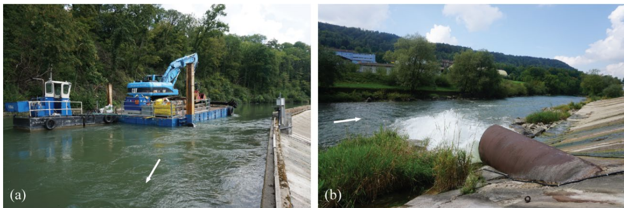
Figure 13: Field calibration on September 4, 2018 with (a) an excavator set up on a float and (b) the outlet of the vortex tube during a calibration run.
