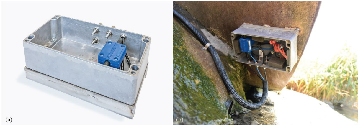
Figure 10: The bedload monitoring setup with (a) the housing and the geophone and (b) the housing mounted to the vortex tube and all sensors installed.
