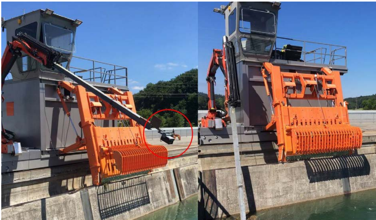
Figure 15: ARIS sonar system at HPP Bannwil. Left: ARIS explorer sonar mounted on an arm of the Palfinger trash rack cleaner. Right: lowered arm with ARIS system in data recording status
