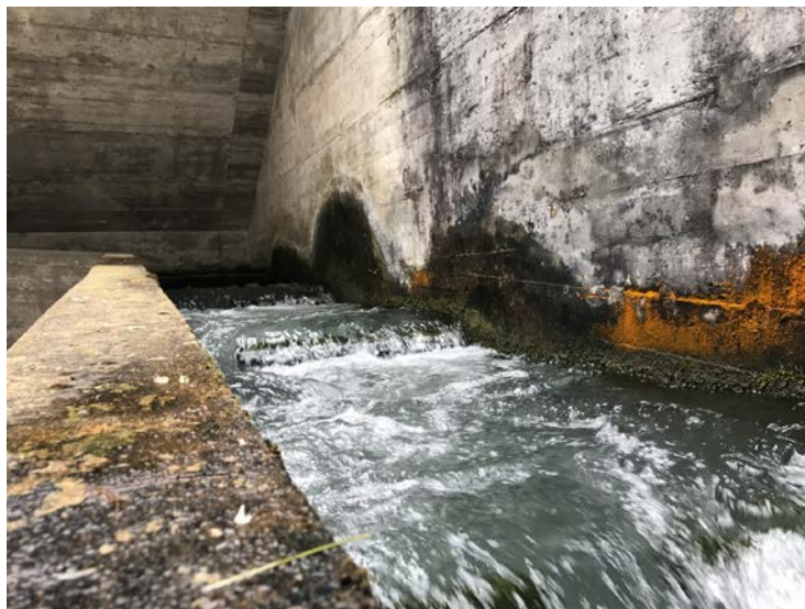
Figure 5: Pool and weir type fish pass with top and bottom openings at HPP Bannwil
