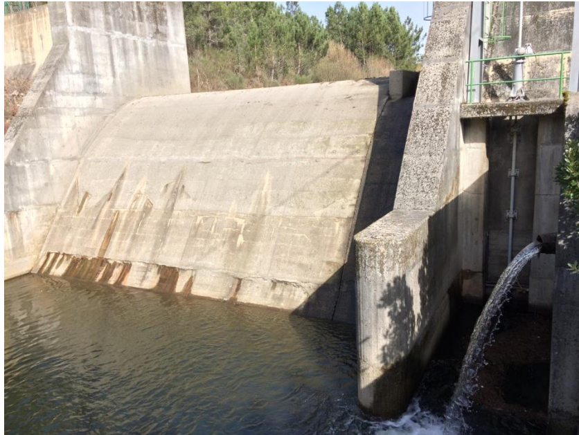
Figure 6 – At the left bank, ecological flow release at the Bragado weir
