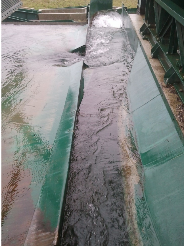
Figure 9: View of the migration duct with an enlargement at the entry of the second outlet
