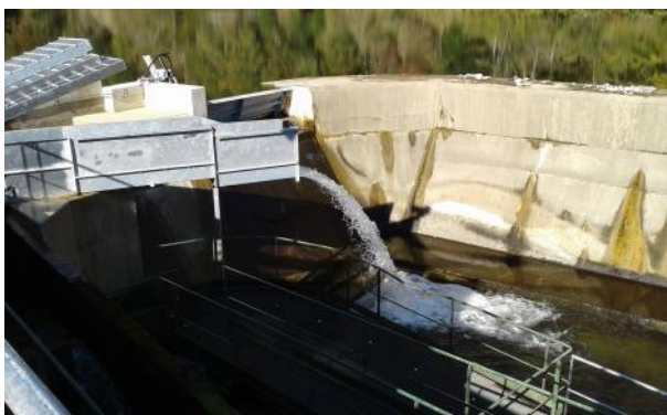
Figure 24: Dump valve on the new weir
