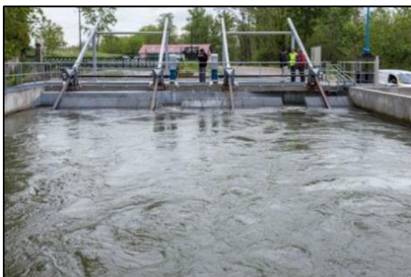
Figure 14: bar screen in water
