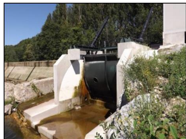
Figure 16: Dump valve for sediments
