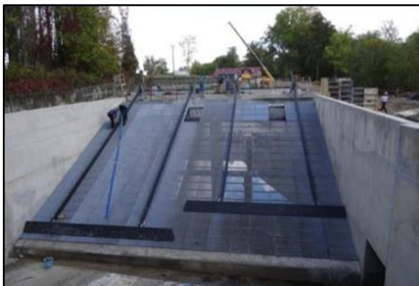
Figure 11: bar screen out of water
