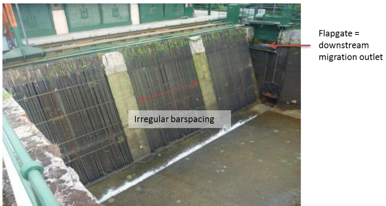
Figure 17: View of the former bar rack at the power plant (source: (Ecogea, 2011))
