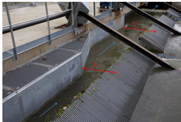
Figure 65: Inclined bar rack and bypass entrances of the Las Rives HPP, with 1st and 2nd gauging sections.
