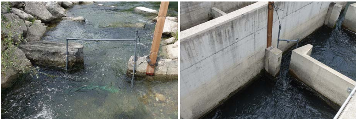
Figure 28: PIT-Tag antennas (left picture in the nature-like fish pass, right picture in the vertical-slot pass)
