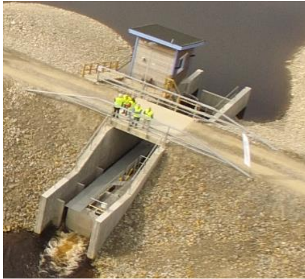
Figure 6: Upstream migration device inlet structure (vertical slot pass with entrance gate)
