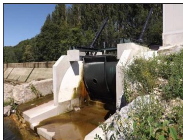
Figure 16: Dump valve for sediments
