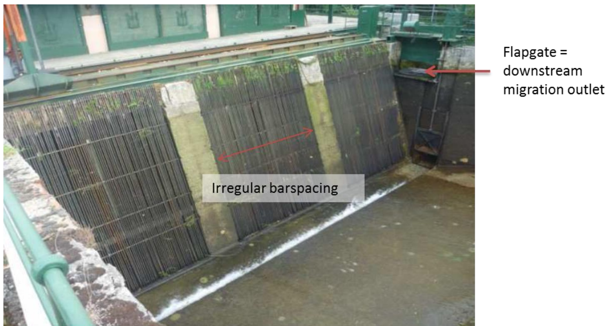
Figure 17: View of the former bar rack at the power plant (source: (Ecogea, 2011))
