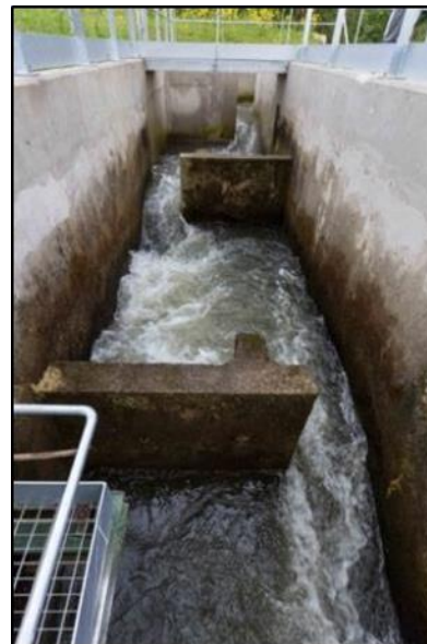
Figure 25: downstream view of the new pools in the fish pass
