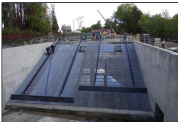
Figure 11: bar screen out of water
