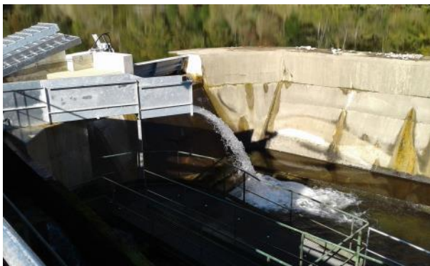
Figure 24: Dump valve on the new weir
