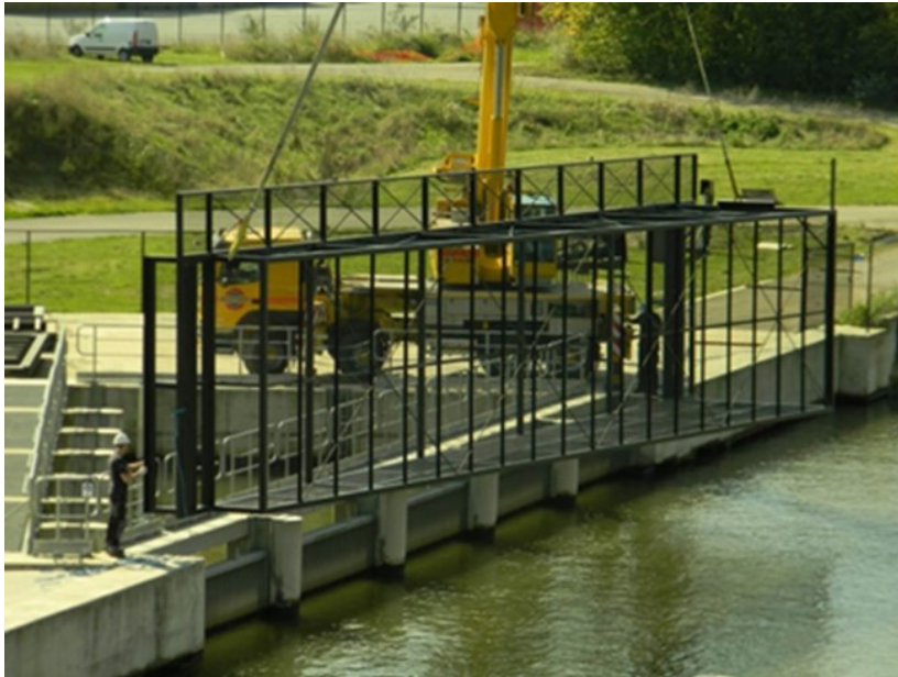
Figure 11 Picture of the installation of the cage to catch tested fish after screw passage (see also Figure 7).
