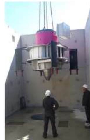
Figure 8: New Dive turbine in the headrace channel (2015) (source: www.dive-turbine.de )
