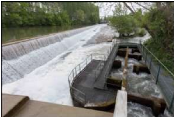
Figure 23: upstream view of the fish pass
