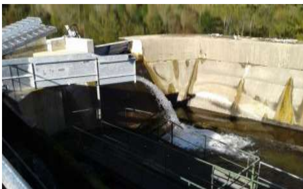
Figure 24: Dump valve on the new weir
