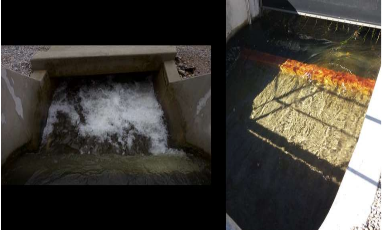
Figure 37: left drop after the control weir until 2017; right: inclined ramp after the control weir today
