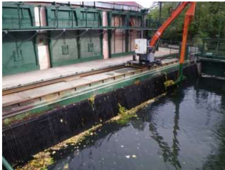
Figure 21: Bar rack in front of the HPP from 2010 to 2014 (Ecogea, 2011)
